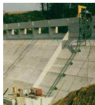
Barrage de Bois Joli (FishPass)
